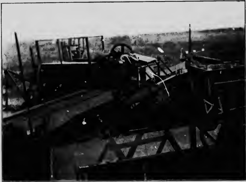
View (seen from above) of Moore's loading hopper, and Anrep's excavator, Alfred, Ontario
